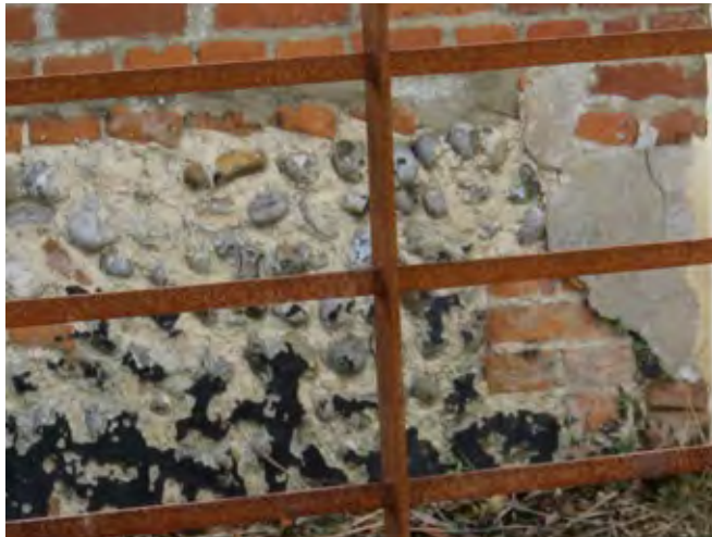
Inappropriate concrete repair
