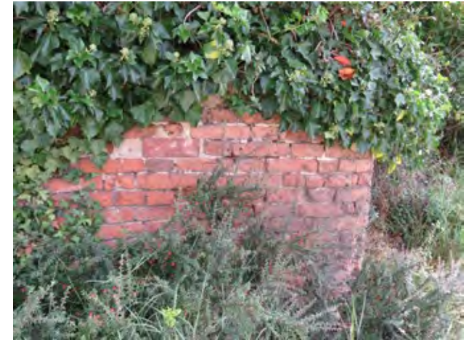
Vegetation growth on brick wall
