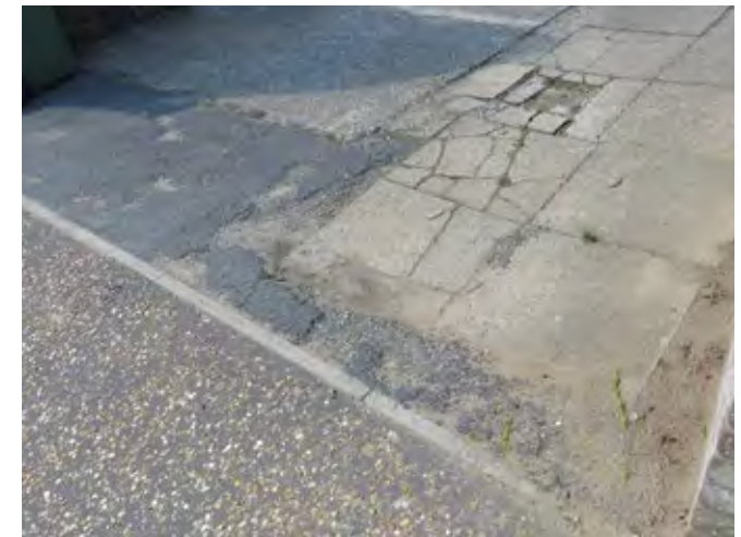
Cracked paving slabs on driveways
