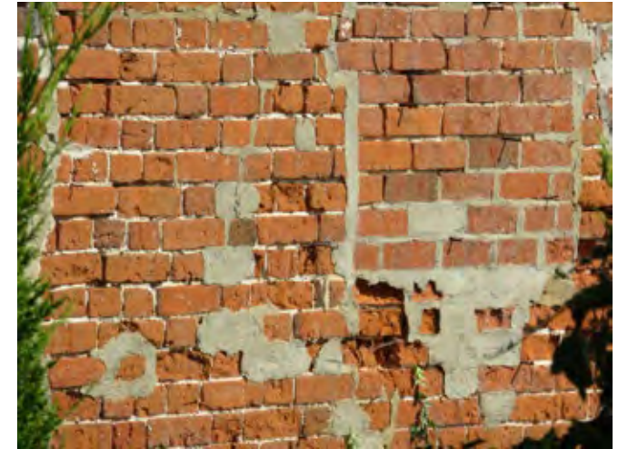
Eroded historic bricks due to cementitious pointing
