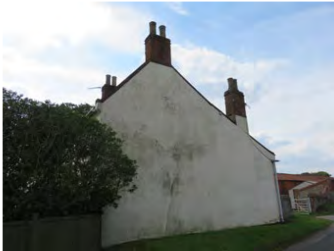
Damp issues seen on external render
