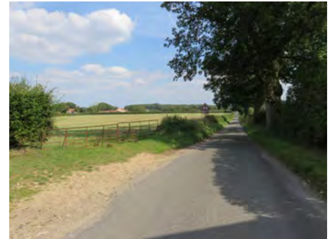
Eroded grass at the edge of the road
